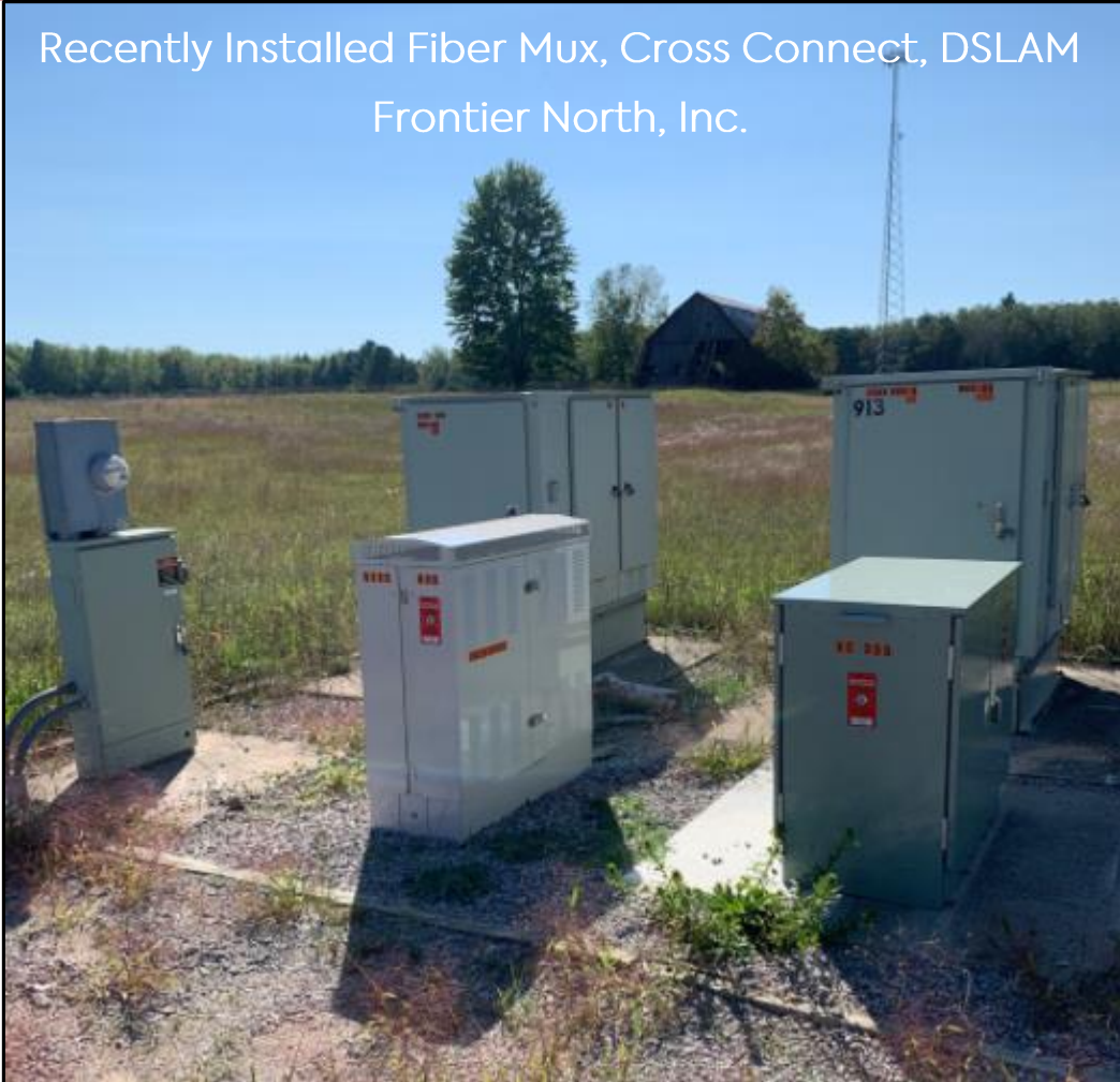
Fiber Optic Vault
